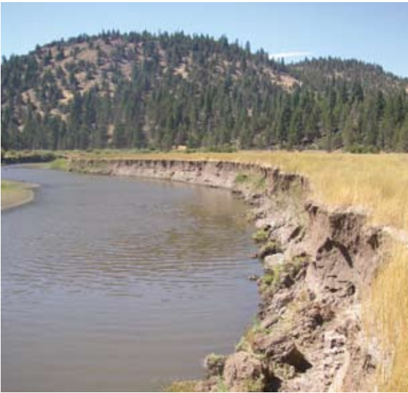
Channel erosion on upper Pit River
