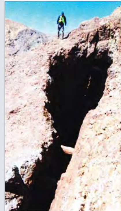
Department of Conservation staff assesses an unmarked mine shaft. Photo courtesy of the California Department of Conservation. LAO
